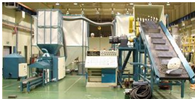
A polystyrene volume-reduction equipment
